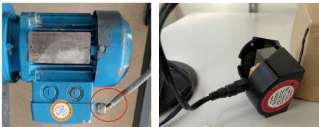
Cable is pulled out and housing is defective: frequently observed defects. Images: E+S.
